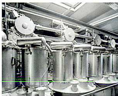
Distribution via diverter valves to internal silos
