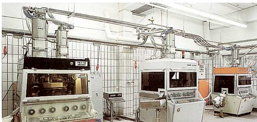
Centralized feeding for several processing machines
