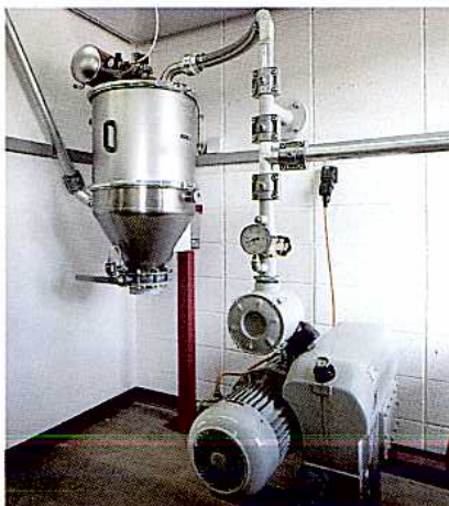
Vacuum pump with upstream secondary filter
