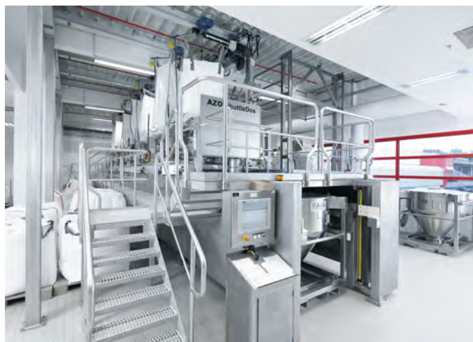
Product feeding level above the dosing and weighing section
