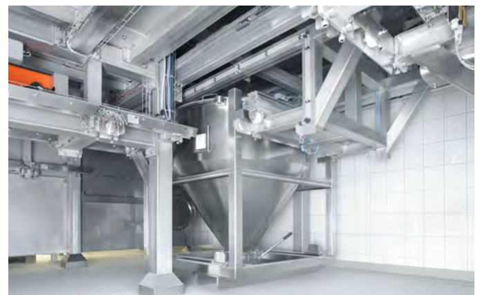
The individual dosing lines are linked with each other by means of cross transport systems
