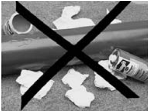
The pipe trench is not a rubbish tip
