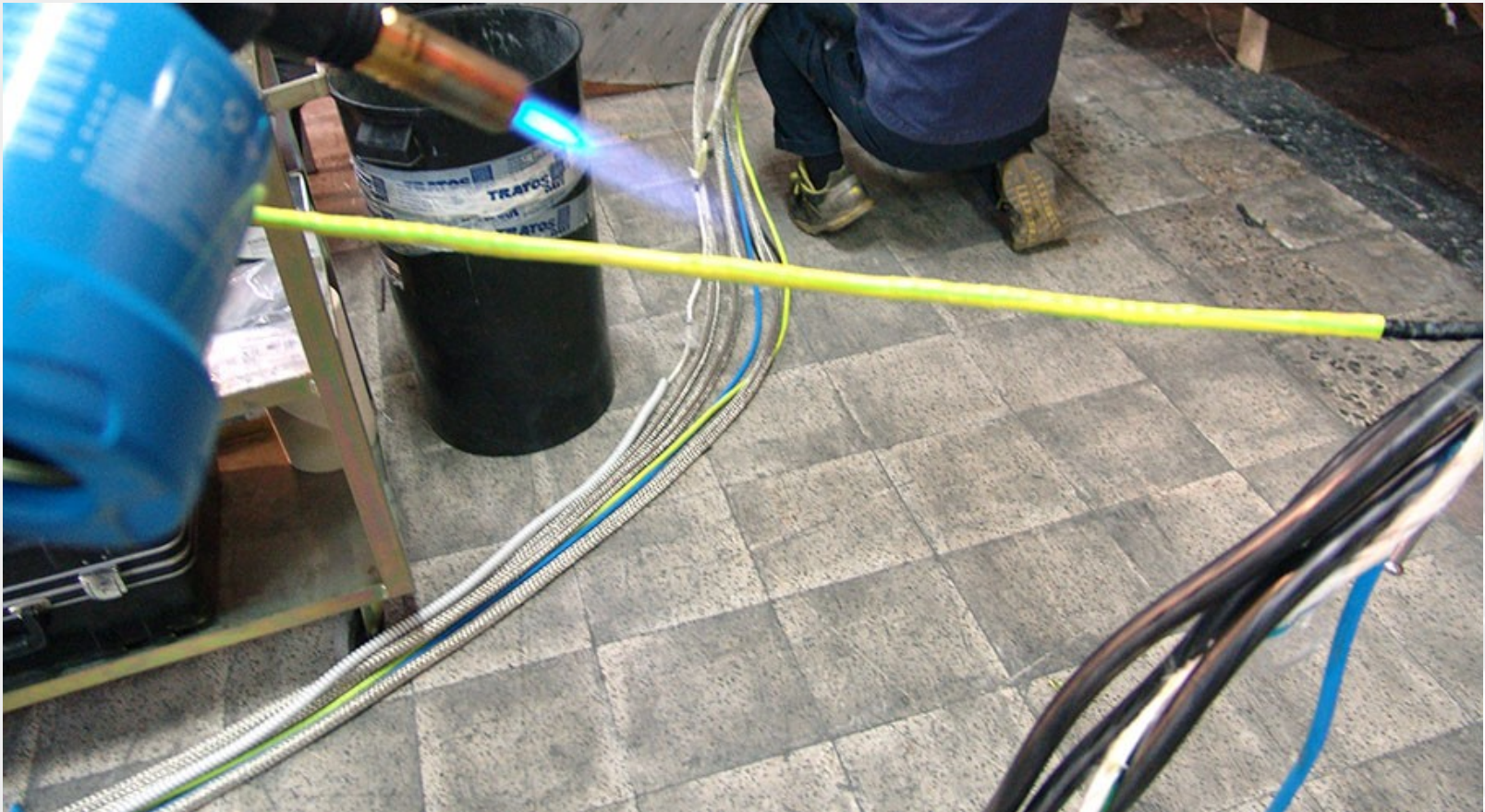
Application of heat shrinkable tube (green/yellow for the Earth and blue for the Ground-Check)
