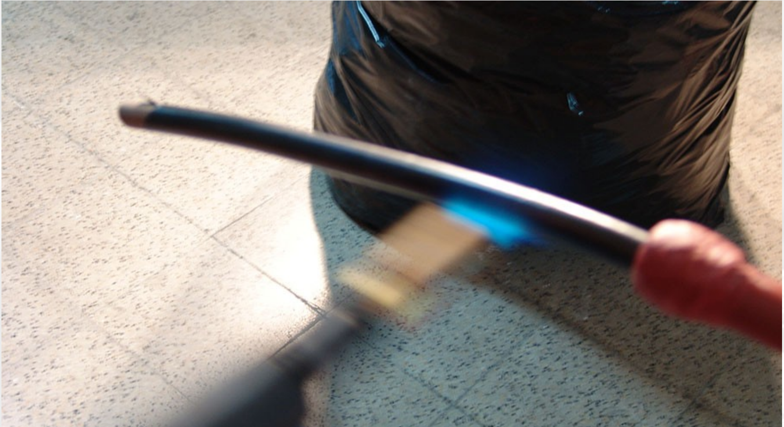
Removal of the external semiconductor in the final part of the Phase
