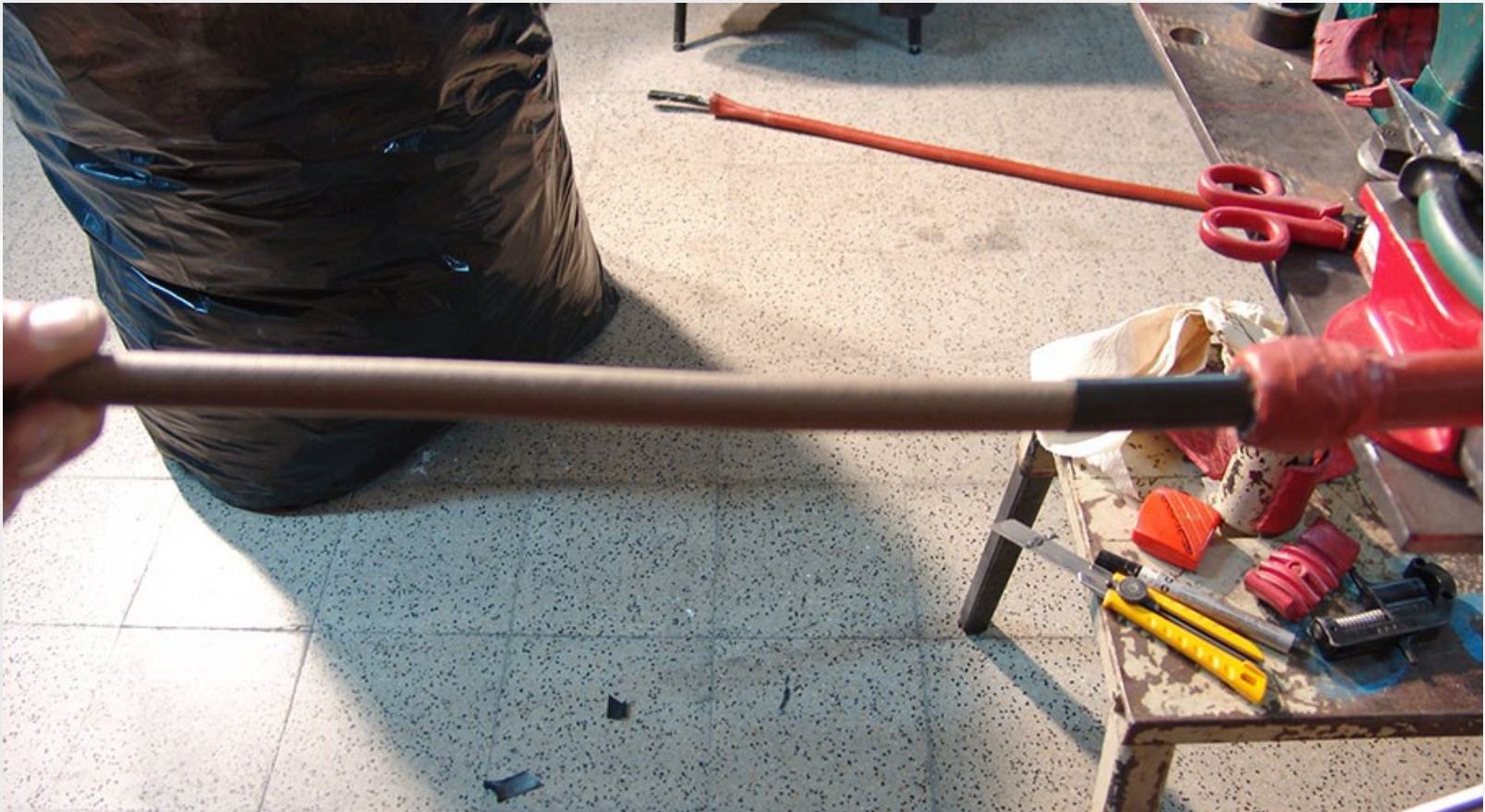
Removal of the external semiconductor in the final part of the Phase
