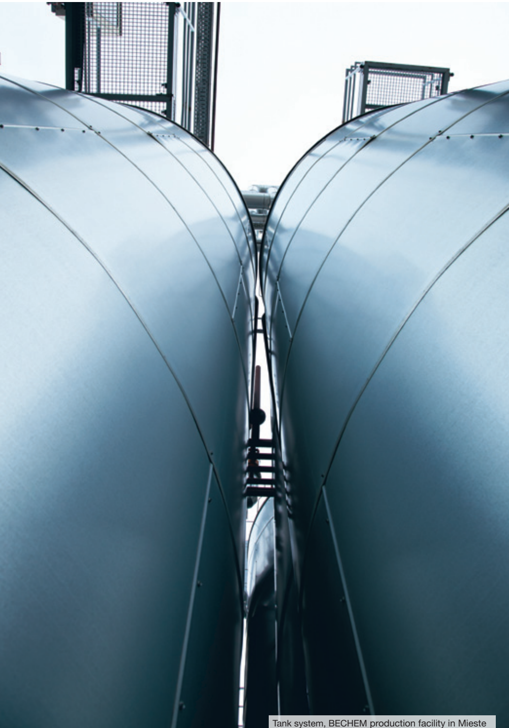
Tank system, BECHEM production facility in Mieste
