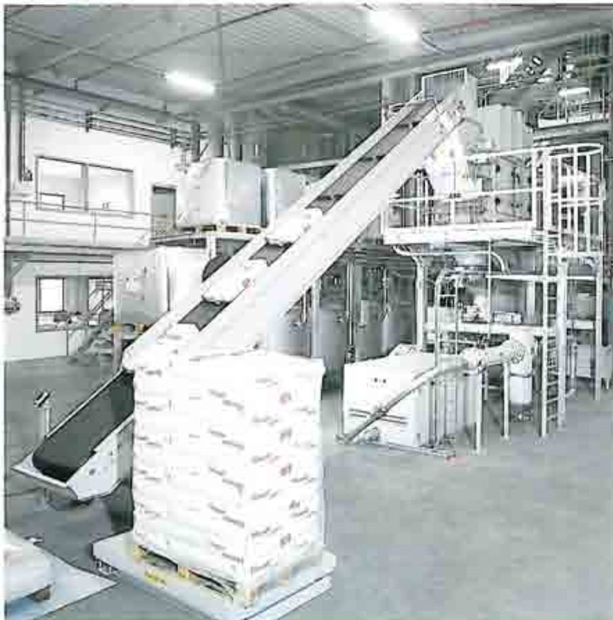
Screens can be used prior to automatic bag filling stations
