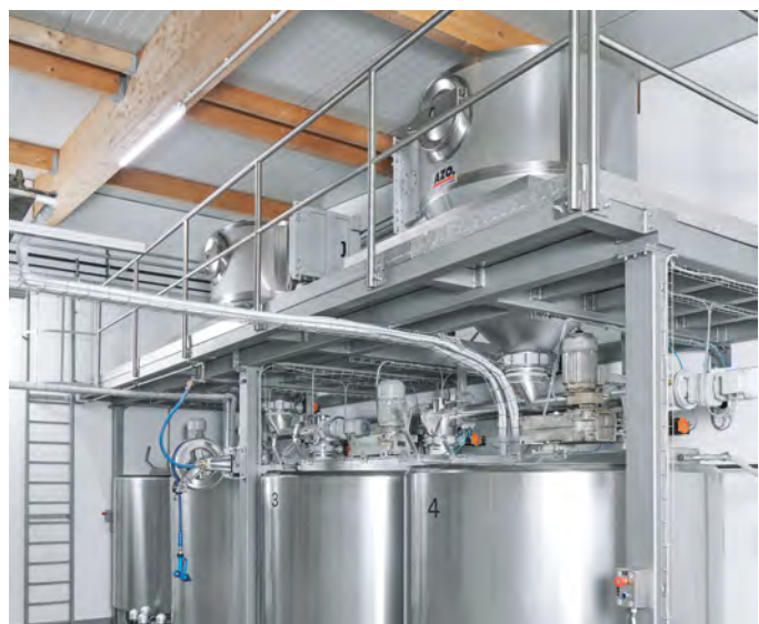
Connecting four batching tanks to the flour supply
