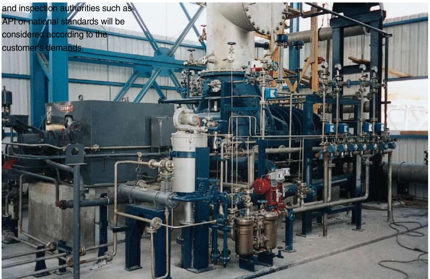
Soda Sanayii, Mersin (Turkey), compression of coke oven gas VRO 836 L, intake volume flow of 45.000 m 3 /h, compression of 0,85 to 3,5 bar (abs.), water-purged carbon labyrinth sealing
