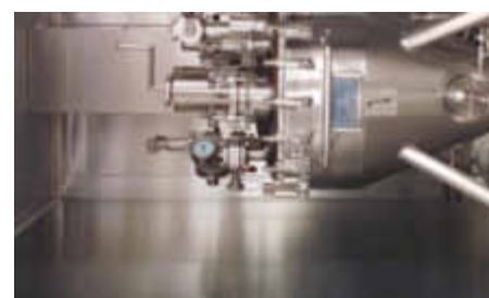
At lifting station for discharge
