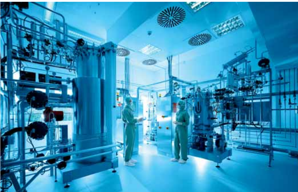
Left: Main production bioreactor, capacity 500 liters. Rear: Inoculum bioreactor, capacity 20 liters. Right: Prefermenter, capacity 100 liters.
